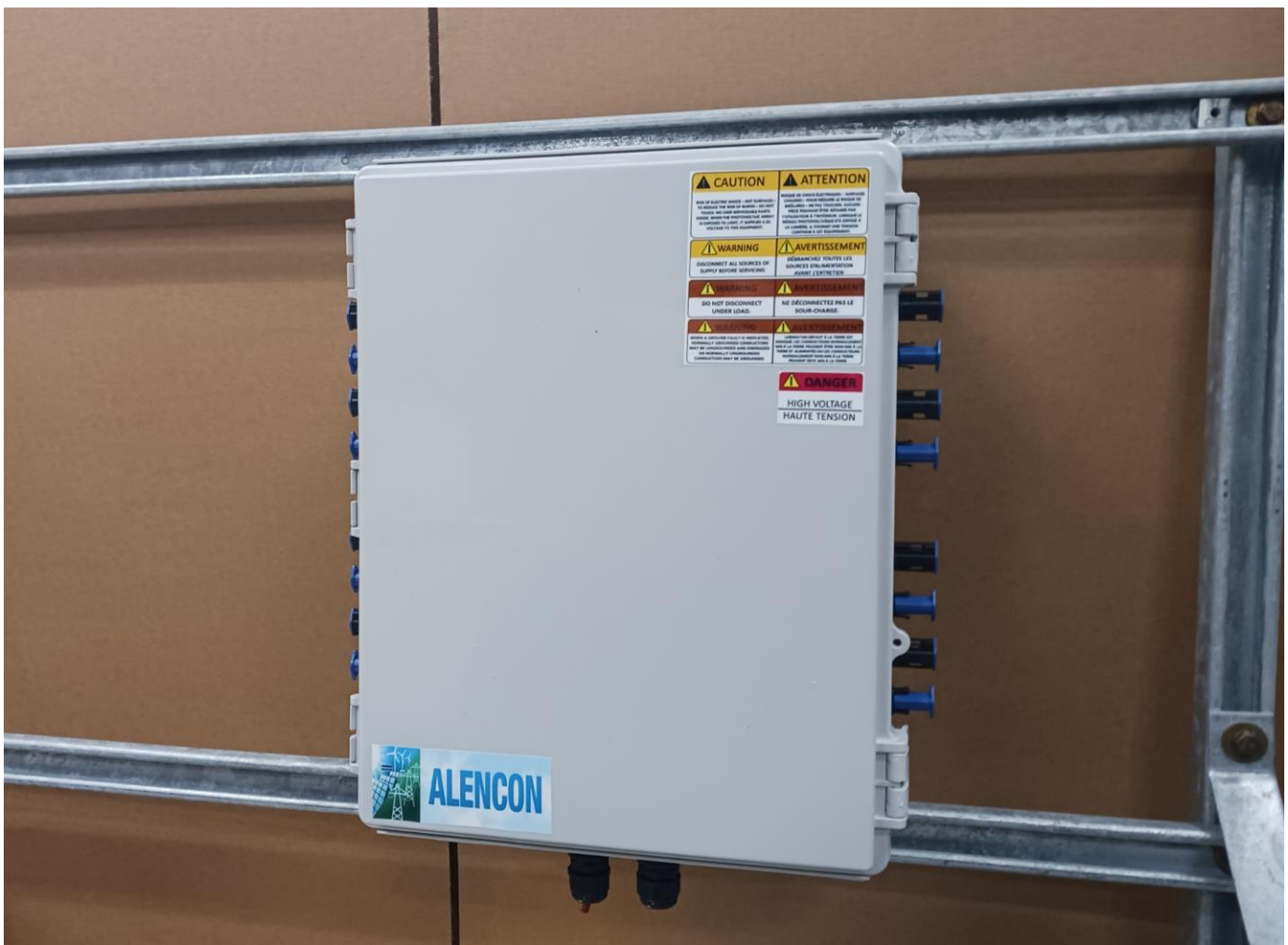
Figure 14: GARD mounted on Unistrut racking
