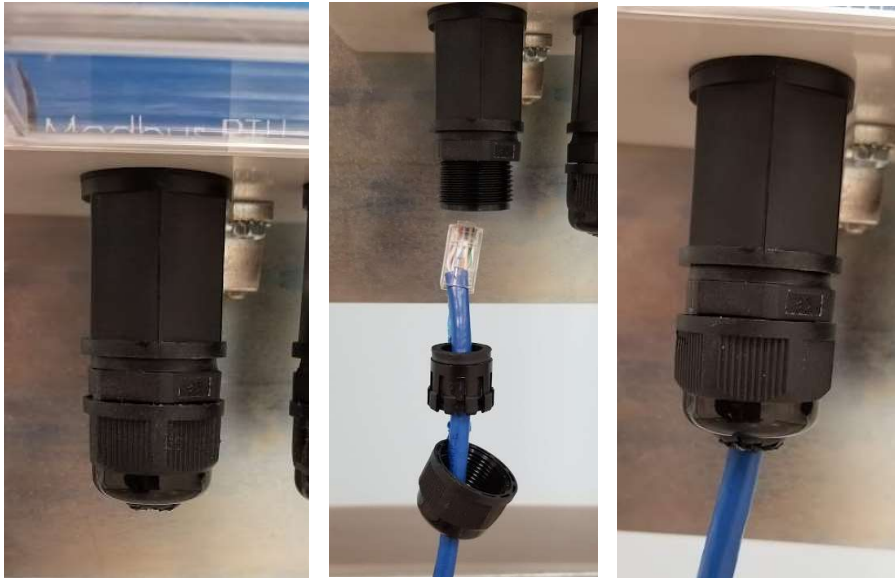
Figure 13: Water-proof wiring on the PODD
