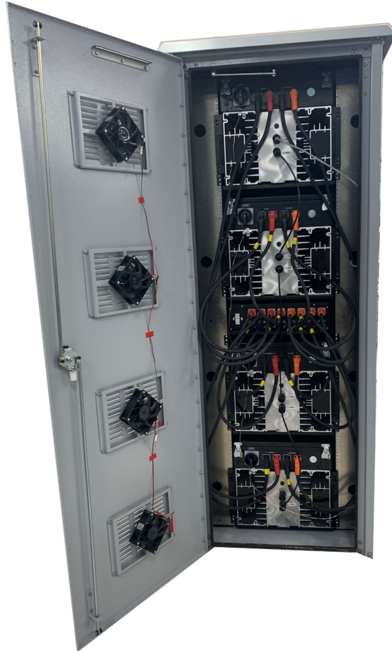
FIGURE 17: BOSS UNITS IN BOX RACKING SYSTEM
