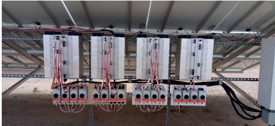
FIGURE 12: SPOTs WITH IMO DISCONNECT
